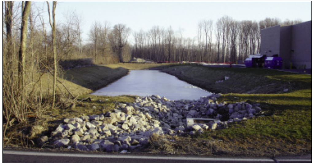
The retention basin and stormwater management facility designed for the Kohl's store provides the required storage while being flexible for future expansion.
