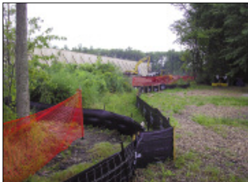
A silt fence was installed along the perimeter of the Lighthouse Village retail development to reduce the amount of sediment flowing into nearby wetlands.
